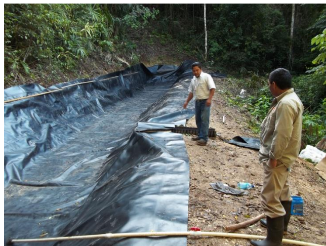
Cleaning Improved Pond at the end of Dry Season - Check for leakage
